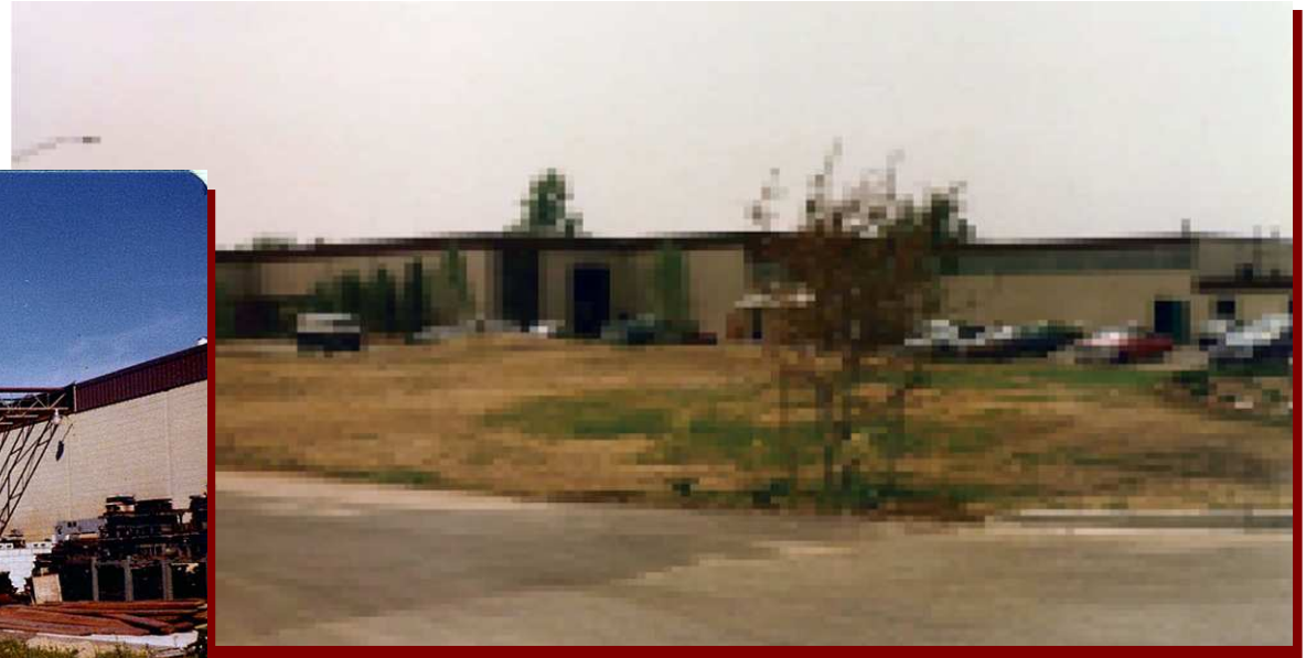
View of the North end of the connection in-between Two existing buildings completed.
