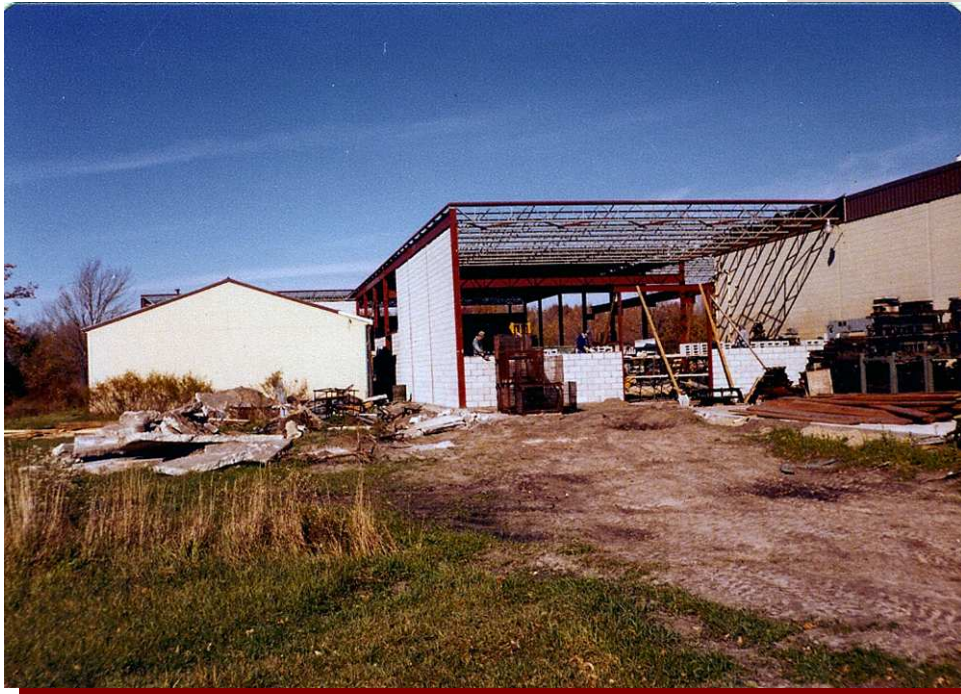
View of the south end of the connection in-between Two existing buildings.
